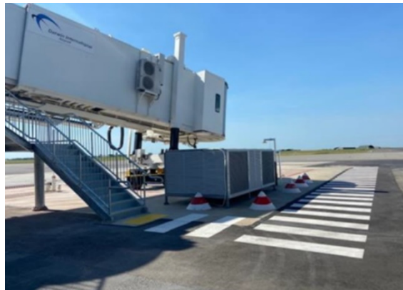
Figure 24: Recently installed preconditioned air unit Bay 2 – November 2021
