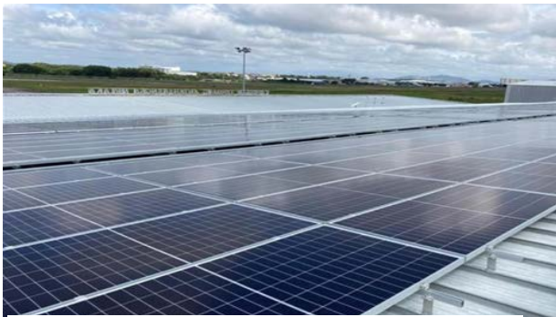
Figure 32: Rooftop Solar, Melaka Airport
