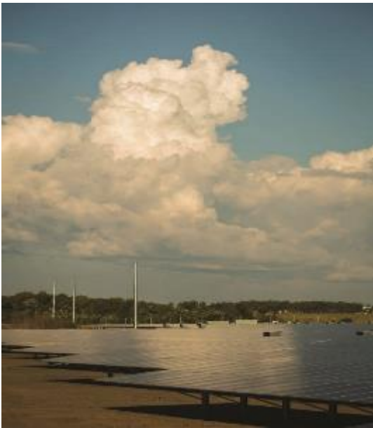
Figure 18: Darwin Airport Solar Project Stage 1
