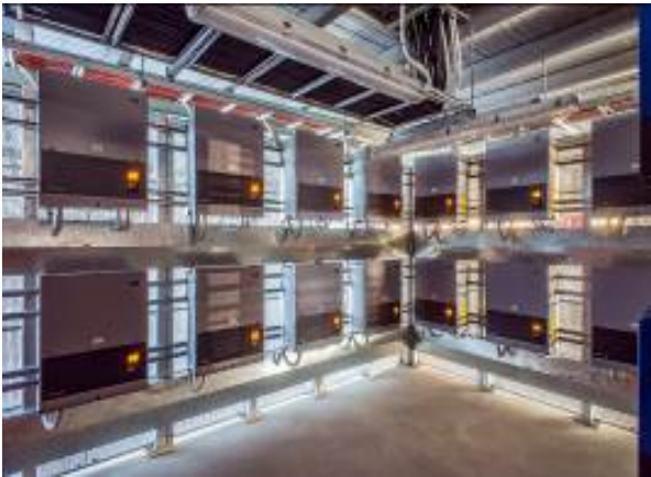
Figure 16: Inverter Room of Adelaide Airport Solar Plant
