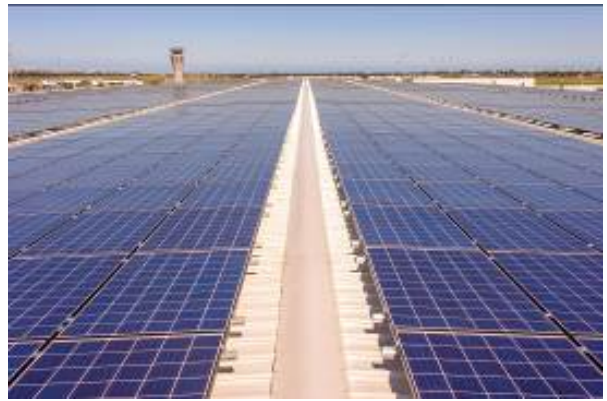
Figure 15: Rooftop View of Adelaide Airport Solar Installation
