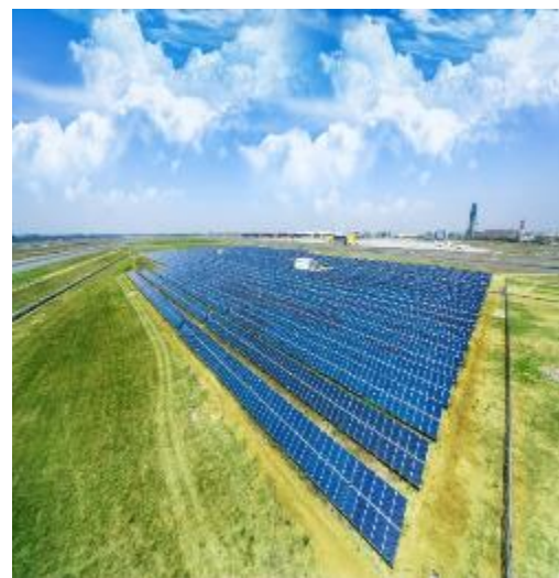
Figure 26: Solar plant of DIAL
