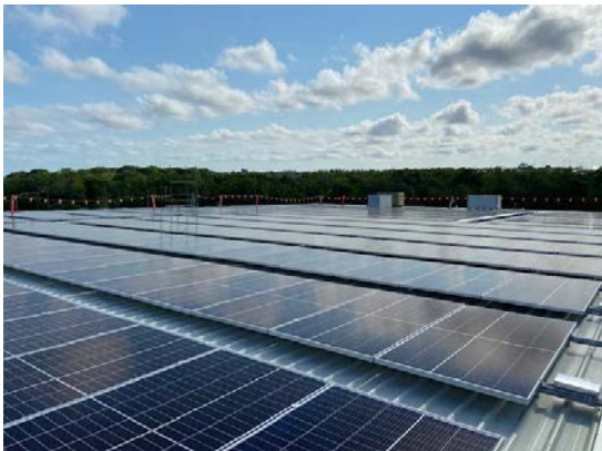
Figure 25: Solar system on cold store Facility 2021
